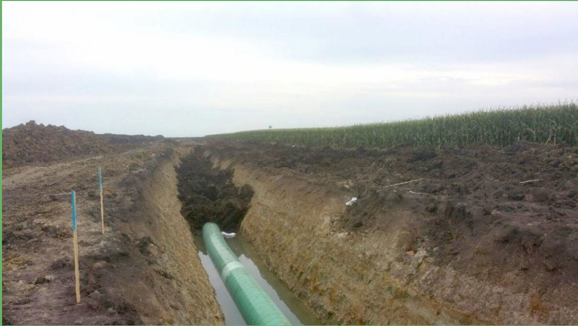
Rich Iowa topsoil at the bottom of the Dakota Access pipeline ditch.
