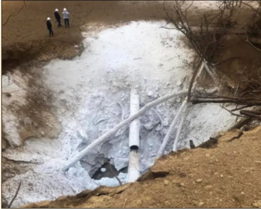
The Satartia pipeline rupture. Source: Yazoo County Emergency Management Agency
